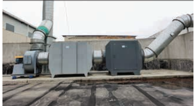
Fu Yu Suzhou – Exhaust Gas Treatment System for Oil Mixing Room and Hazardous Waste Warehouse (completed in 2019)
